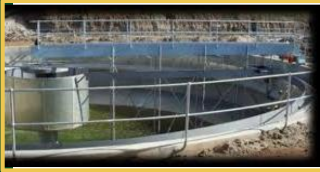
Figure 13: Conventional Settling Tanks ( Ares Tank Clarifier Tank )
