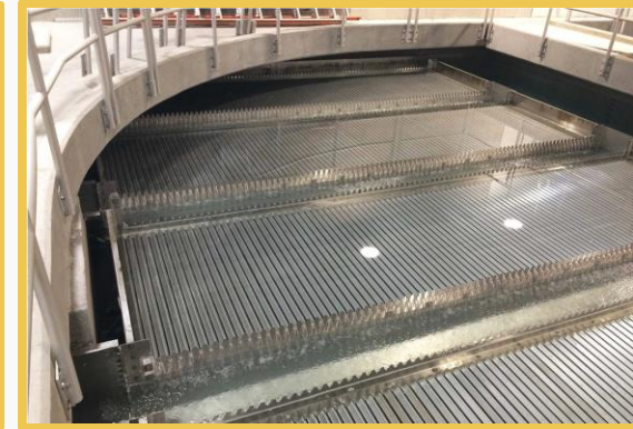
Figure 15: Plate Settlers ( Jim Myer & Sons INC Plate Settler System )
