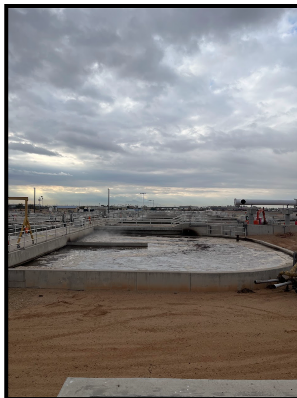
Photo 4: Plant 3 Oxidation Ditch
